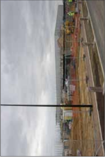
View looking south towards the Barrett Homes development from the central spine road
